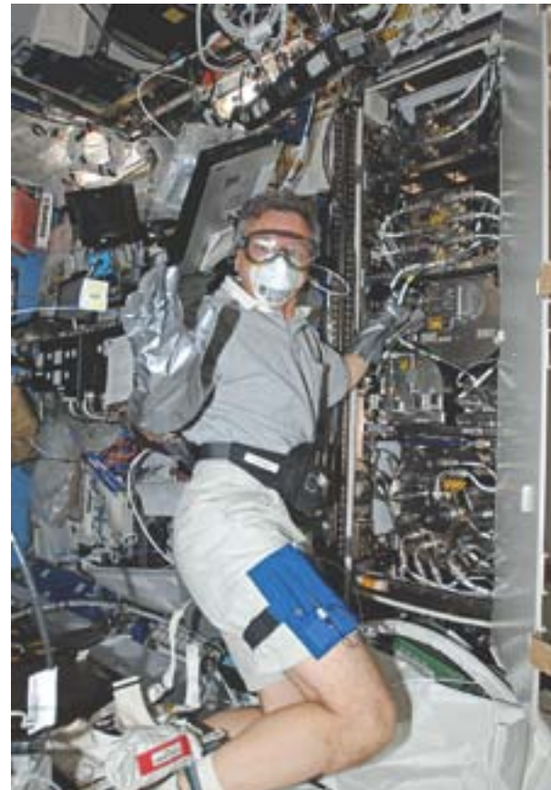
Figure 2: Robert Thirsk, MDCM, performs maintenance on the Station's Water Recovery System. This recycling system processes waste water and crew urine into potable water.
