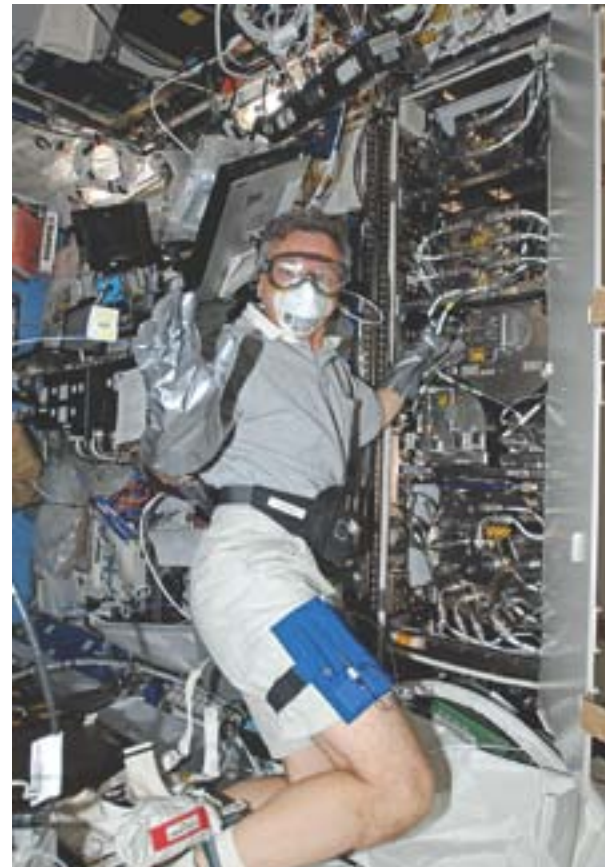
Figure 2: Robert Thirsk, MDCM, performs maintenance on the Station's Water Recovery System. This recycling system processes waste water and crew urine into potable water.
